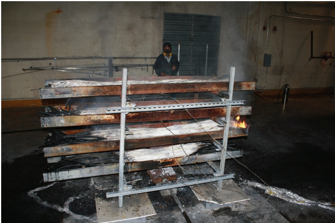
Figure 8-15. Damage to cables following Multiple Tray Test 14.
