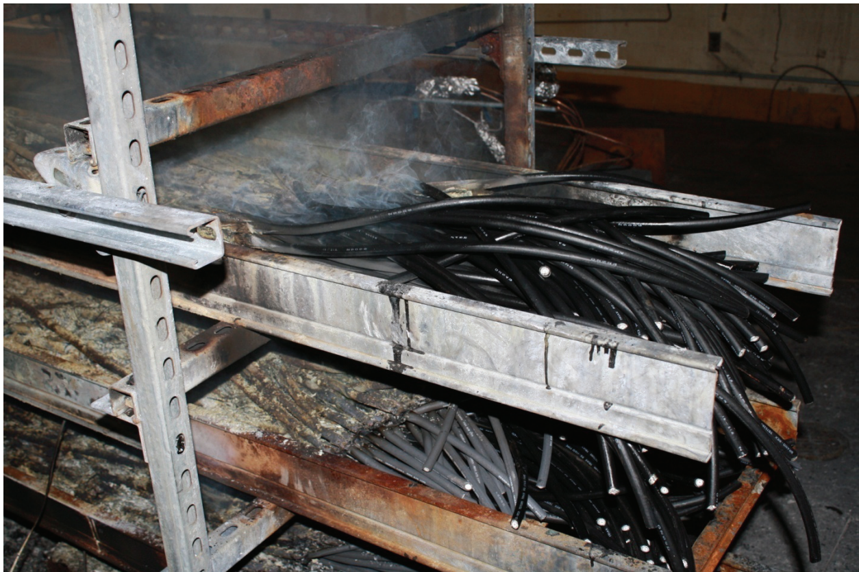
Figure 8-19. Damage to cables, Multiple Tray Test 16.
