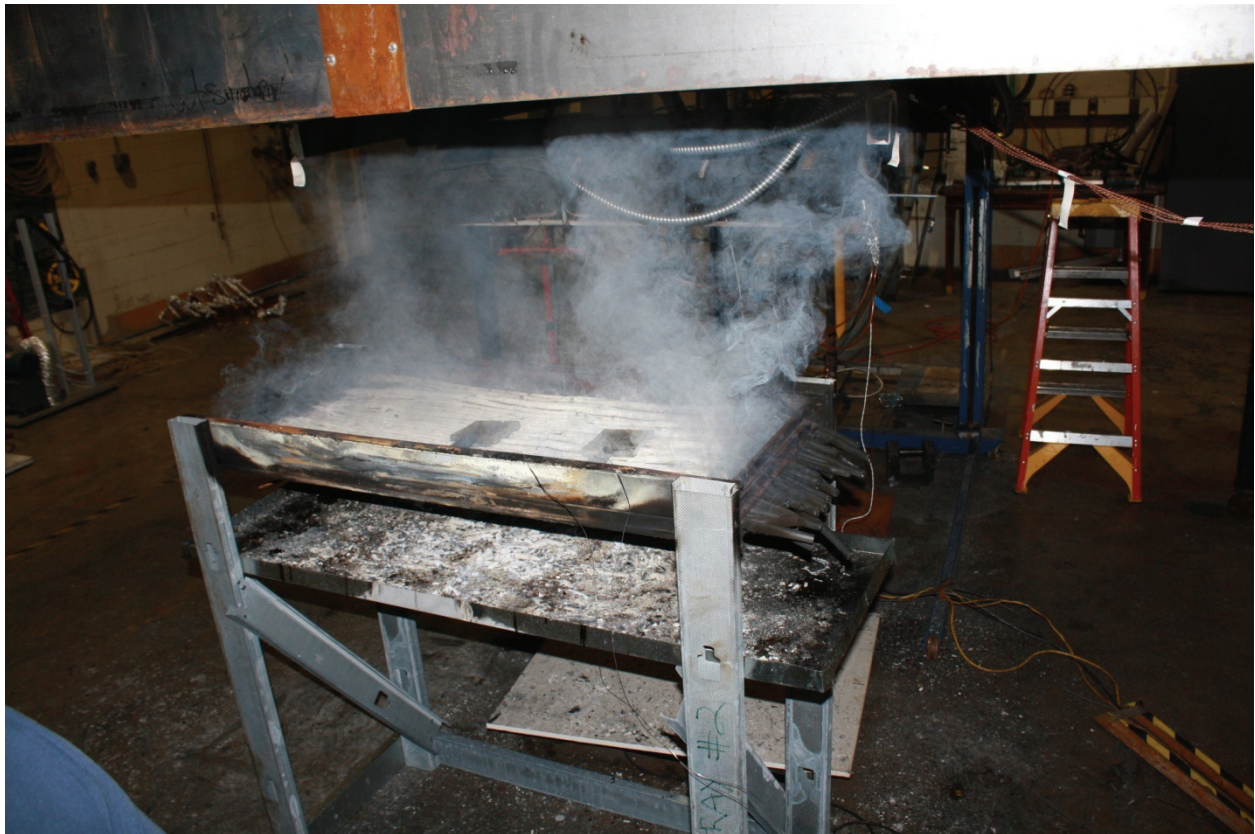
Figure 7-10. Photograph of the remains of the cables in RP-24.
