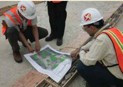
NRC staff participates in site inspection of the proposed new plant in Levy County.
