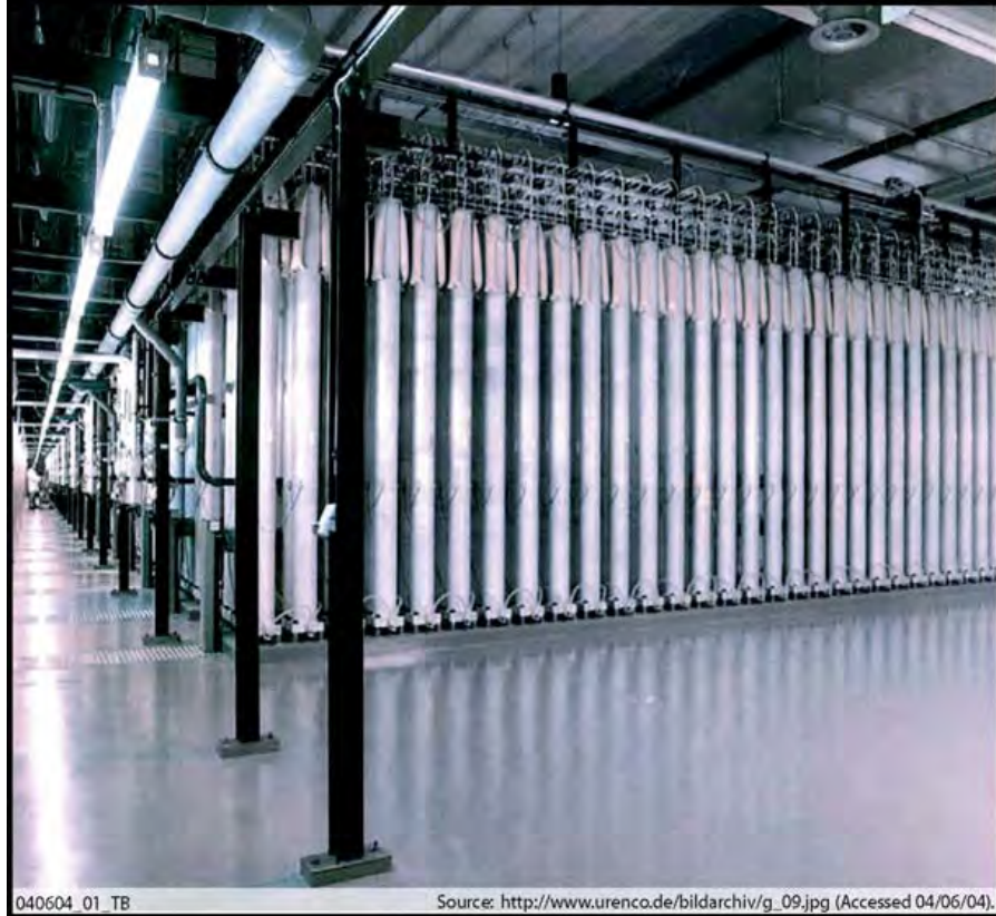
1 2 Figure 2-5 Centrifuges inside a Cascade Hall (NRC, 2005b)
