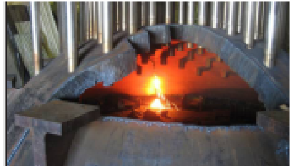
Sectioning of reactor vessel head penetrations from Washington Nuclear Power, Unit 1, a canceled plant
