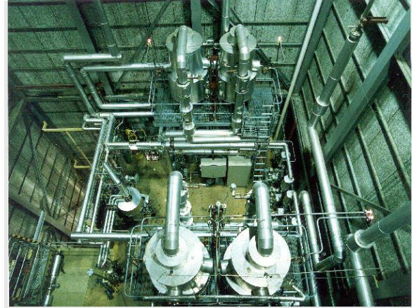
Upper View of the Primärkreislauf-Versuchsanlage (primary coolant loop test facility) PKL Test Facility in Erlangen, Germany
