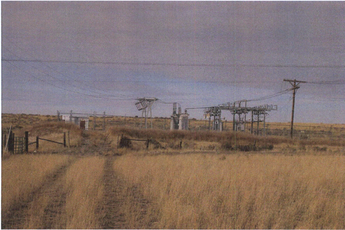
Figure H-5c. Kettle Substation, facing west.
