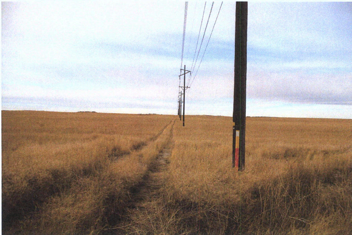
Figure H-5d. Existing 69-kV transmission line along route from Bonneville Substation to the Kettle Substation,
