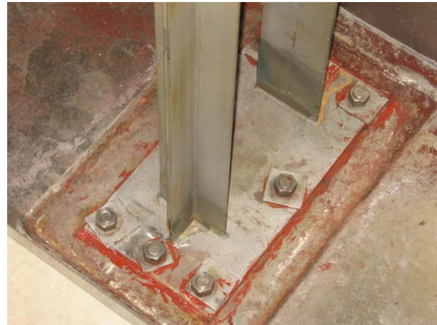
Typical RCCA Change Fixture Support
