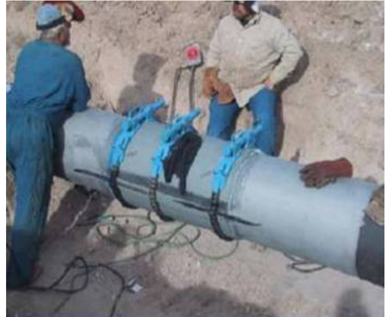
Welded Leak Box
