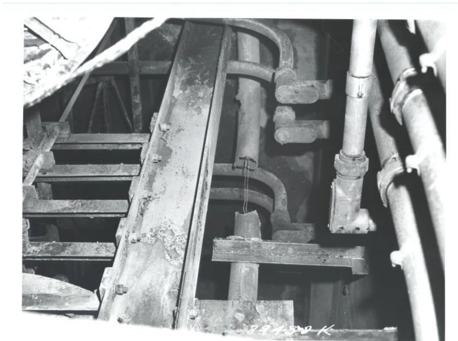
Figure A-1. Photograph of Conduit Damaged from Fire
