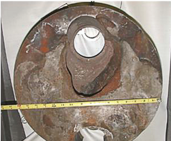
Figure 2. Region of the vessel head depicted by the model and photo of the cavity after it was removed from the vessel head
