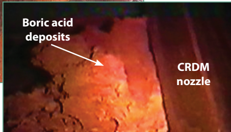
Figure 3b. Boric acid deposits accumulating near a CRDM nozzle (still photo of video taken during the 2000 refueling outage at DBNPS)
