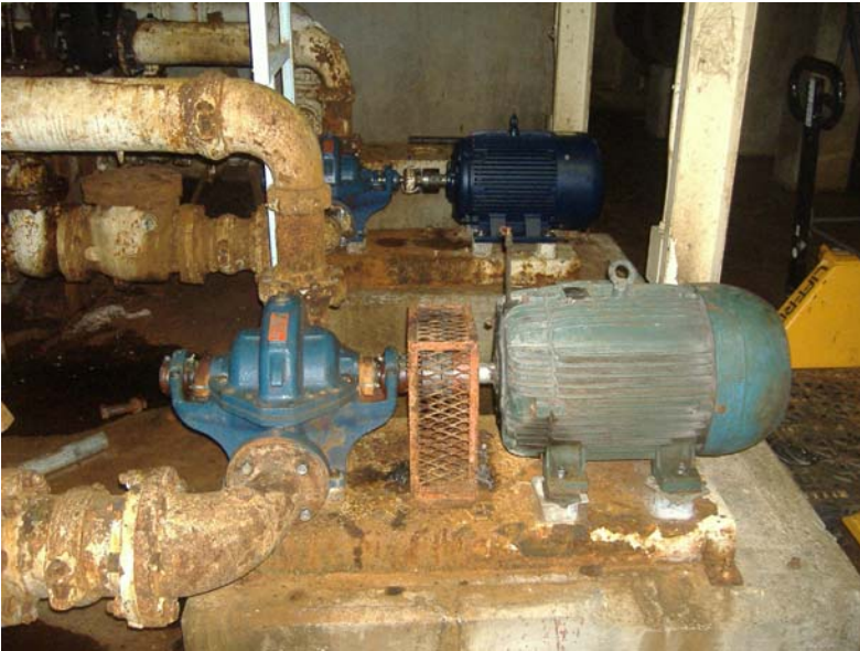
Figure 1: Pump 1 – front Pump 2 - background
