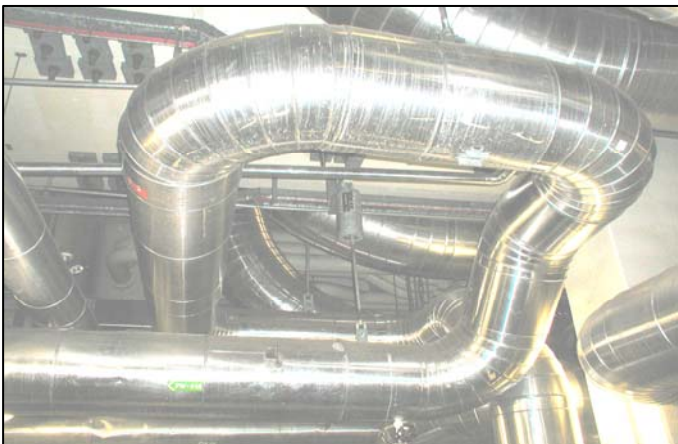
Figure 7. Piping Geometry with Combination of Elbows Upstream of the Location of the UFM Transducer
