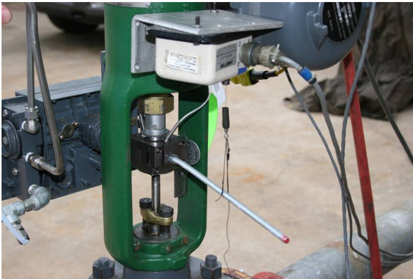
b) The Crane ForceLink used to measure thrust and LVDT used to measure stem travel
