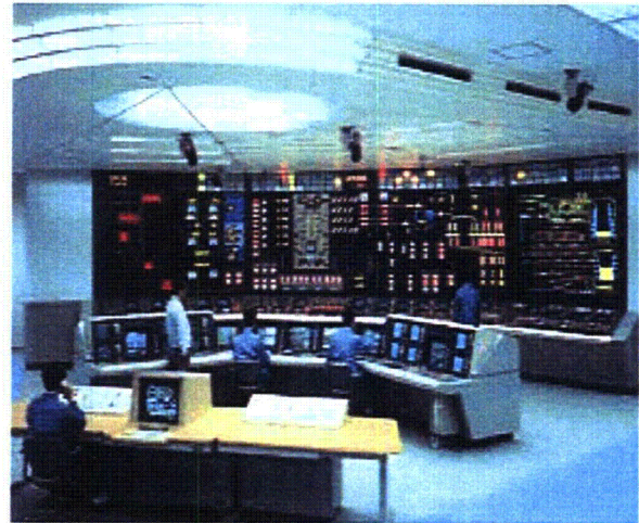
A Highly Integrated Control Room
