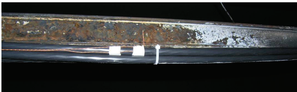
Figure 6.64: Photograph of the horizontal air-drop cable bundle from IT-11.
