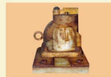
GAUGE WITH OXIDATION
