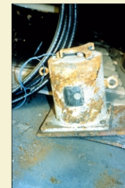
GAUGE PAINTED OVER
