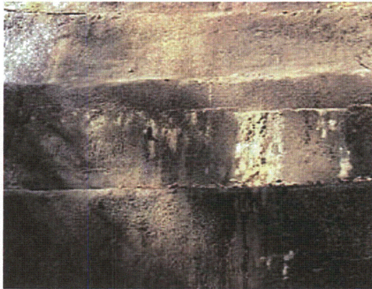
Figure 4.10 Efflorescence in water structure.
