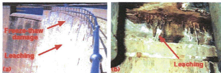
Figure 4.12 Examples of leaching of concrete: (a) dam with freeze-thaw damage and leaching, (b) nuclear power plant tendon gallery leaching.
