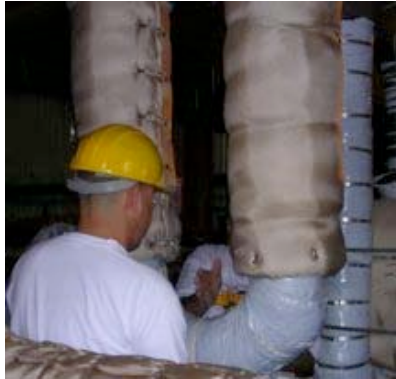
#69: Outer insulation on cable air drop.
