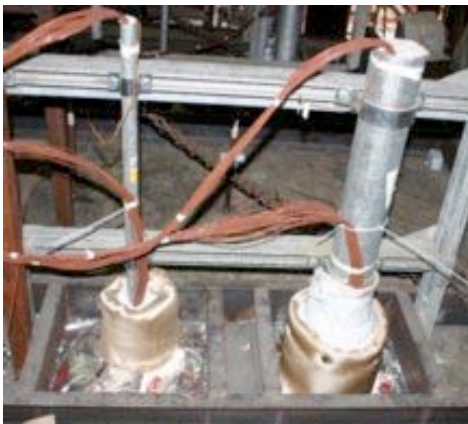
#87: Typical seal on cold side.
