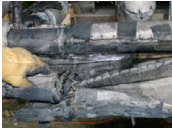
#136: Conduit blackened inside 3C.
