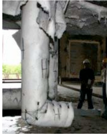
#122: Item 3H after hose stream test.
