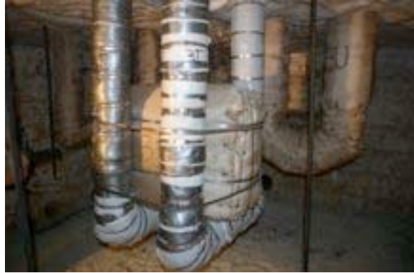
#86: Item 3I in furnace.
