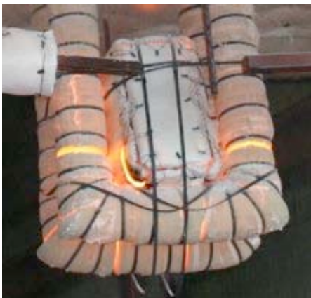
#101: Item 3I junction box.
