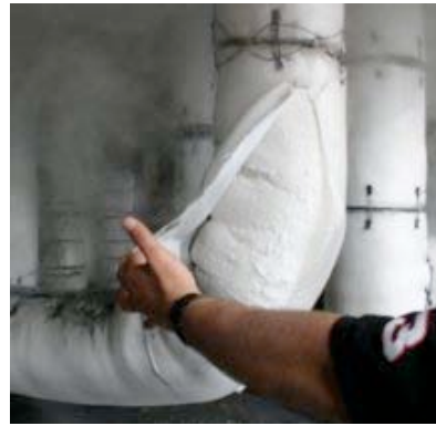
#112: Torn siltemp on 3D.
