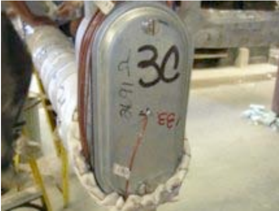
#25: LB cover on conduit 3C.
