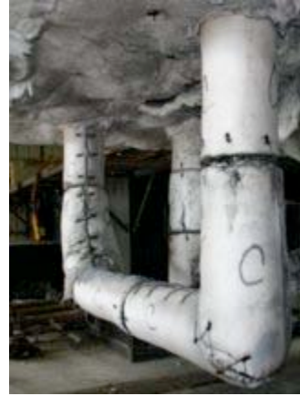
#116: Item 3C after hose stream test.
