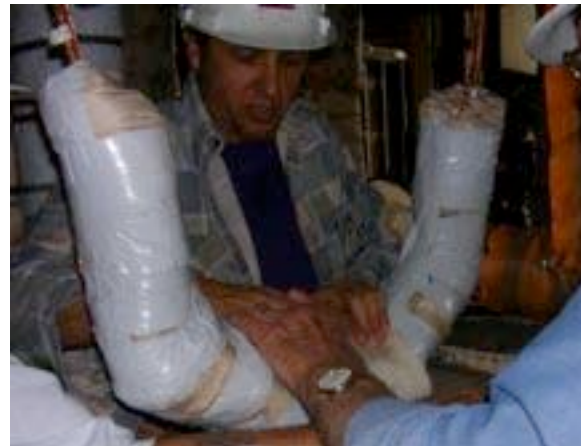
#64: Inner insulation on cable air drop.
