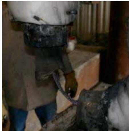
#137: Cable air drop blackened.
