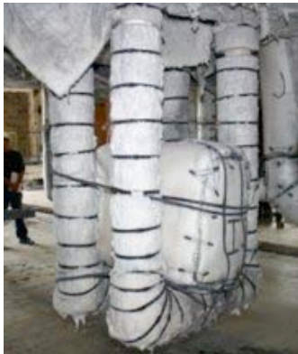
#123: Item 3I junction box after hose stream test.
