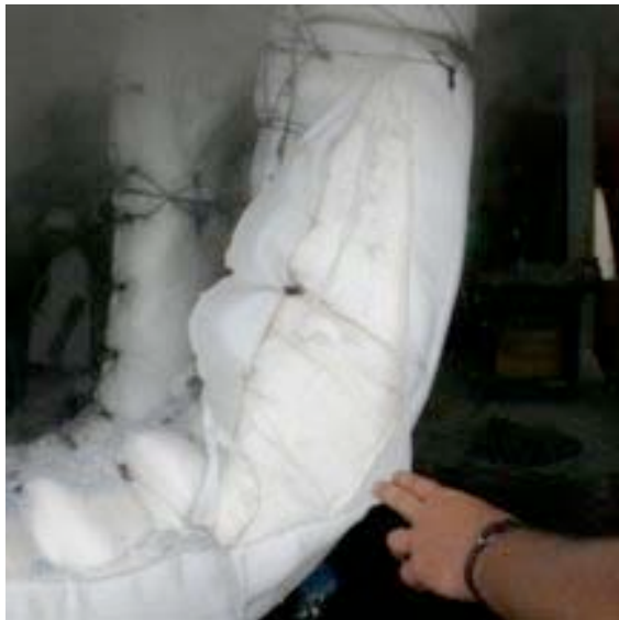
#113: Torn siltemp on 3B.
