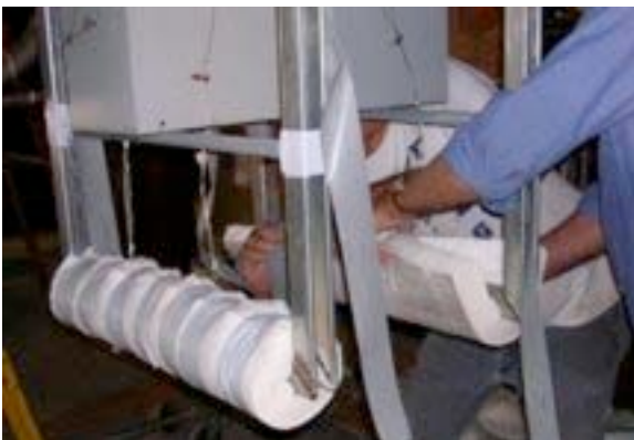
#53: Supports on 3I junction box.
