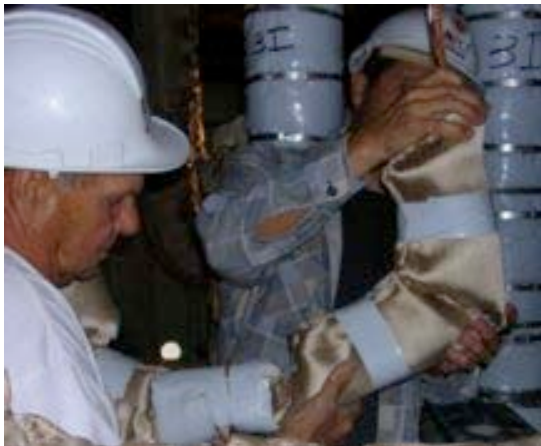
#63: Inner insulation on cable air drop.
