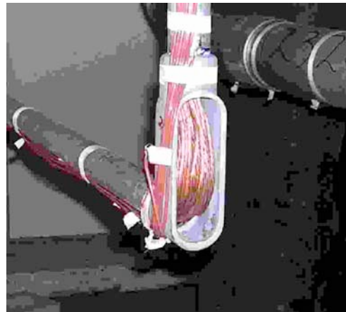
#6: Conduit with bare #8 inside.
