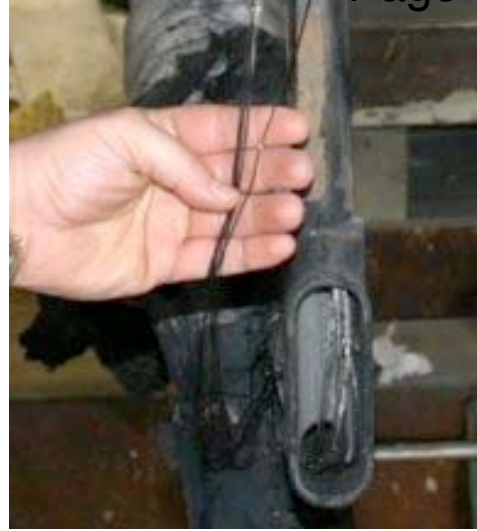
#134: 3E TC wires are burned bare.
