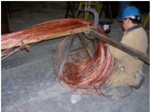
#5: Wire bundle for 4" conduit.
