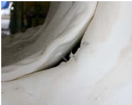
#125: Bolt loose on 2D inside elbow.
