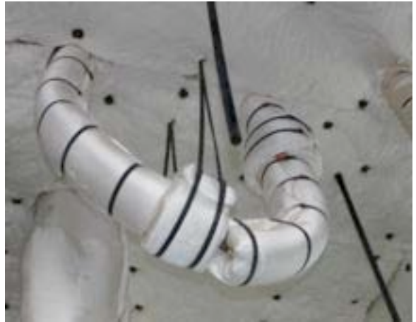
#100: Item 2F after fire exposure.
