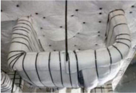
#109: Item 2C with opening after hose.
