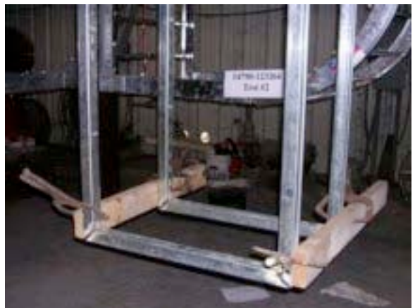
#10: Junction box supports.
