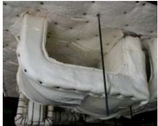
#112: Item 2D after hose stream test.
