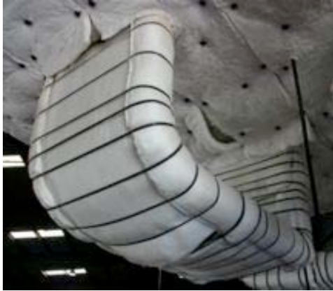
#115: Item 2C after hose stream.
