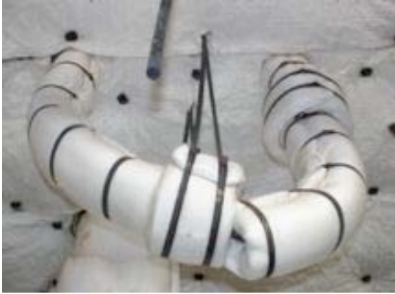
#121: Item 2F after hose stream.
