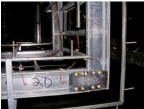
#9: 2" air gap on item 2D.
