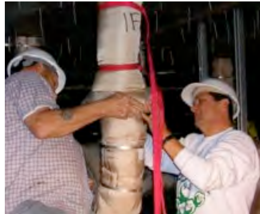
#46: Cladding overlap on conduit 1F.
