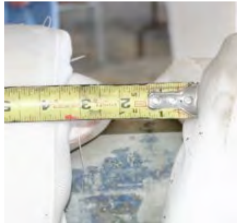
#136: 2.5" gap in conduit 1A after collar was removed.
