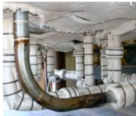
#138: Conduit 1A with insulation off.
