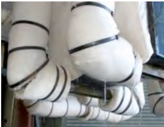
#131: JB supports after hose stream.
