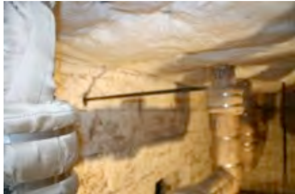
#82: Typical furnace TC.
