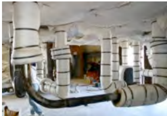
#144: Conduit 1C with insulation off.
