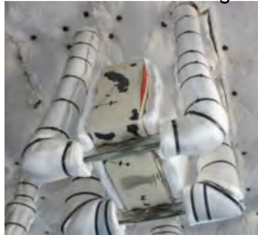
110: Junction box hot.
