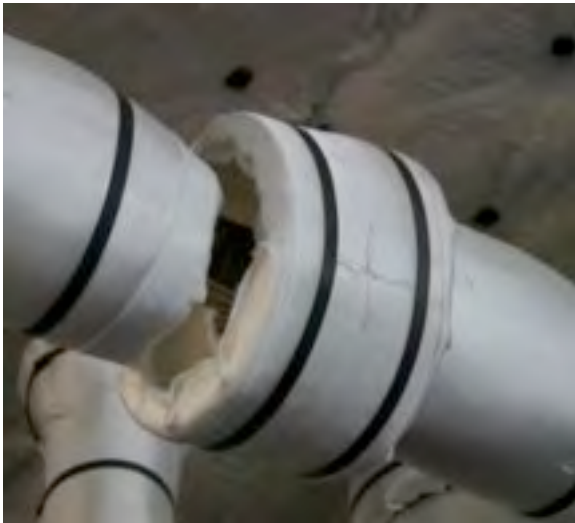
#107: Opening in conduit 1D.
