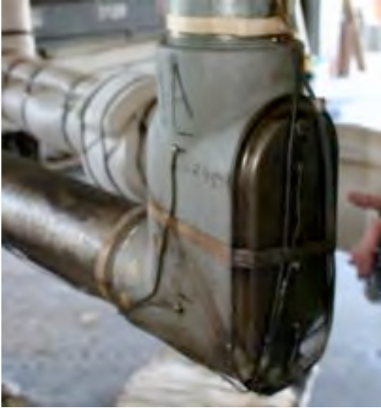
#139: Conduit 1A LB with insulation off.
