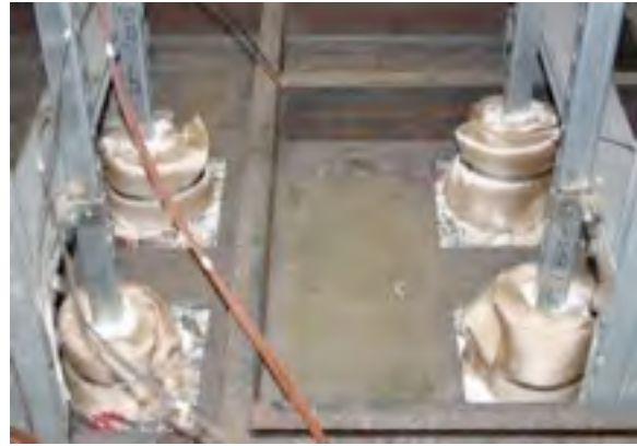
#94: Top side, junction box.
