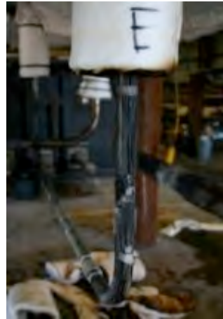
#148: Conduit 1E with insulation removed.
