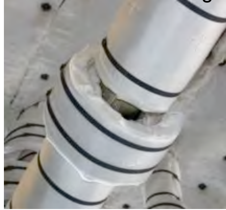
#104: Gap in conduit 1A insulation.
