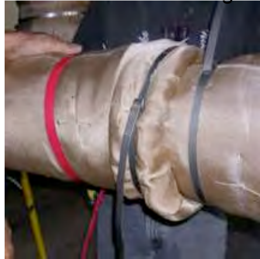
#38: Banding overlap on conduit 1C.
