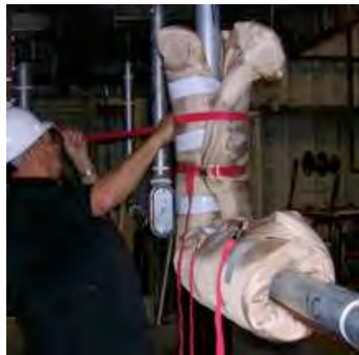
#36: Cladding LB on conduit 1C.
