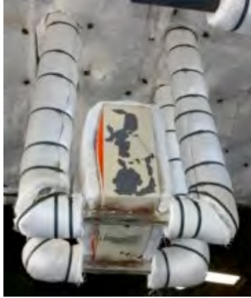
#103: Junction box still hot.
