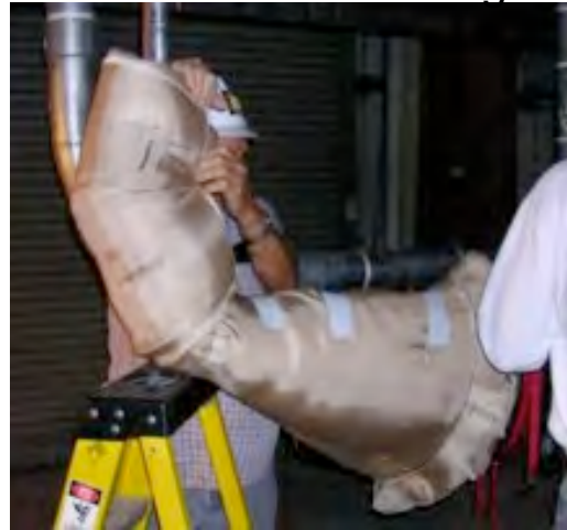
#44: Cladding elbow on conduit 1F.
