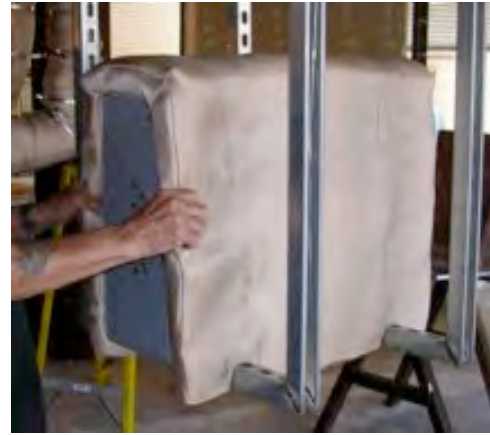
#52: Cladding Junction Box.
