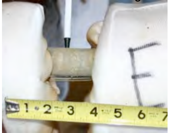
#146: Conduit 1E with collar removed.
