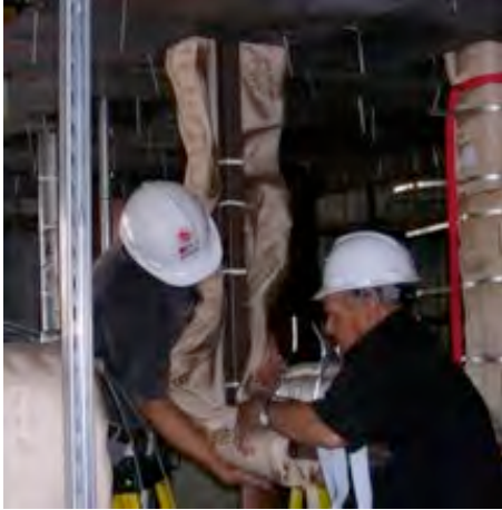
#49: Cladding support 1H.
