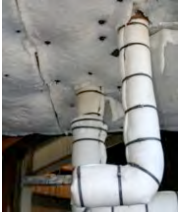
#127: Item 1G after hose stream.
