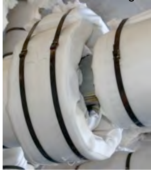
#140: Open joint on conduit 1B.
