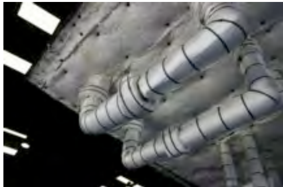
#102: Gap in conduit 1A.
