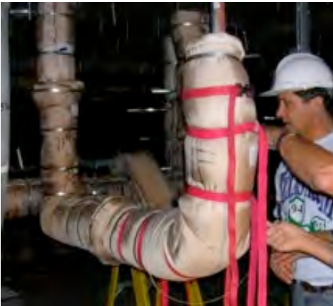
#45: Cladding elbow on conduit 1F.
