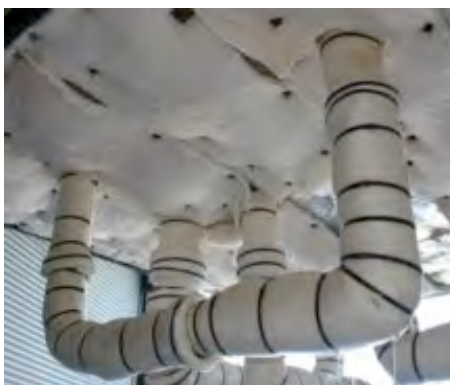
#125: Item 1C after hose stream.
