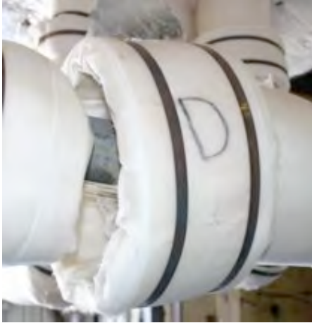
#145: Open joint in conduit 1D.
