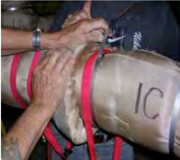
#37: Cladding overlap on conduit 1C.
