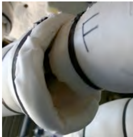
#149: Open overlap joint on 1F.
