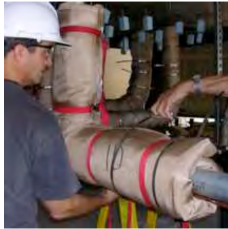
#40: Cladding LB on conduit 1D.
