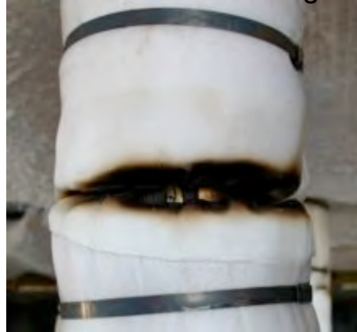
#134: Conduit 1A with collar removed.
