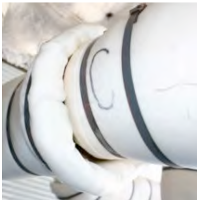
#143: Gap in conduit 1C.
