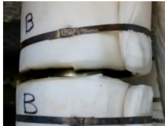
#142: Gap under collar on conduit 1B.
