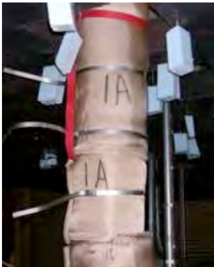
#29: Joint on conduit 1A.
