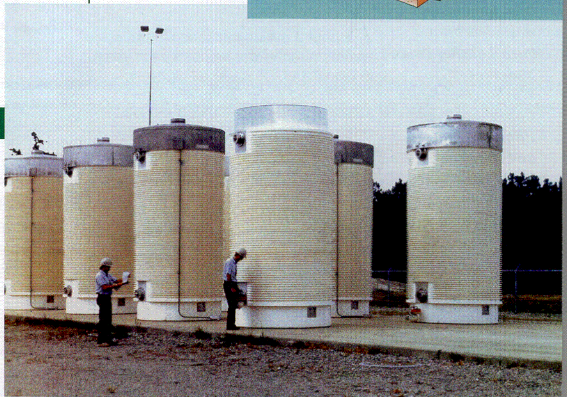
Storage casks at the Surry Nuclear Power Plant in Virginia
