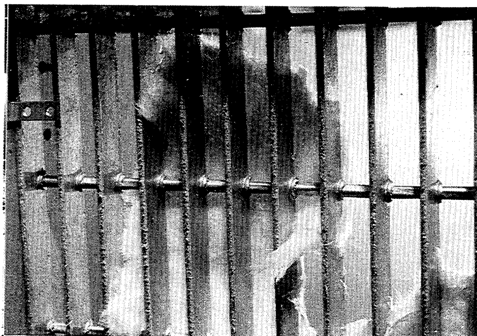
B) VIEW FROM DOWNSTREAM; THE INSULATION EDGES WRAPPED AROUND AND THROUGH THE BARS
